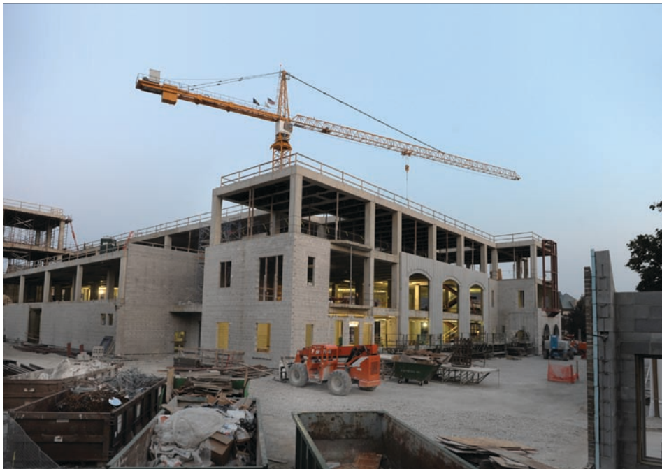
Early view of the new Stinson-Remick engineering facility, a 142,000-square-foot facility that will house a nanotechnology research center, the University's new Energy Center, an 11,800-square-foot semiconductor processing and device fabrication clean room, and an undergraduate interdisciplinary learning center.
